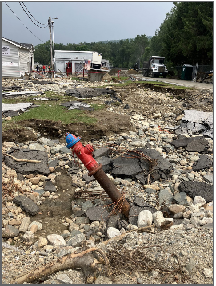
Ludlow Wastewater Treatment Flood Damage, 2023
