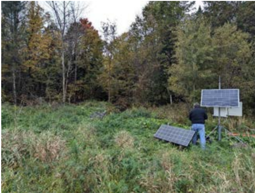
Lake Carmi tile drain filter study site 4. Lower solar panels are located at the filter inlet and outlet.
