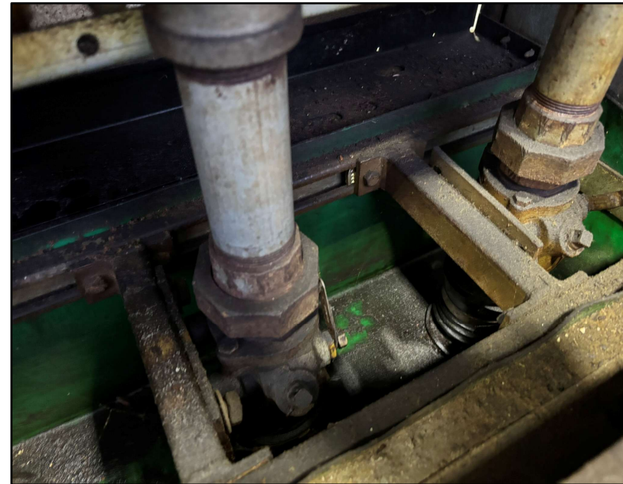
Solid debris and trace amounts of fuel in dispenser sump
