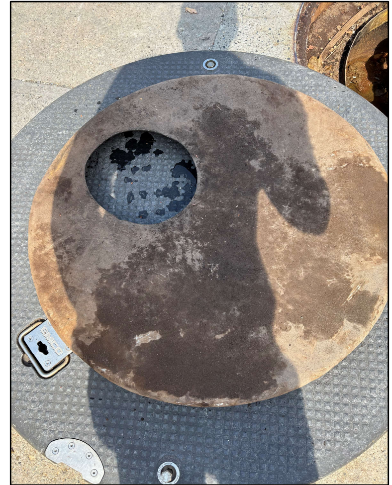
Hole in turbine sump covers
