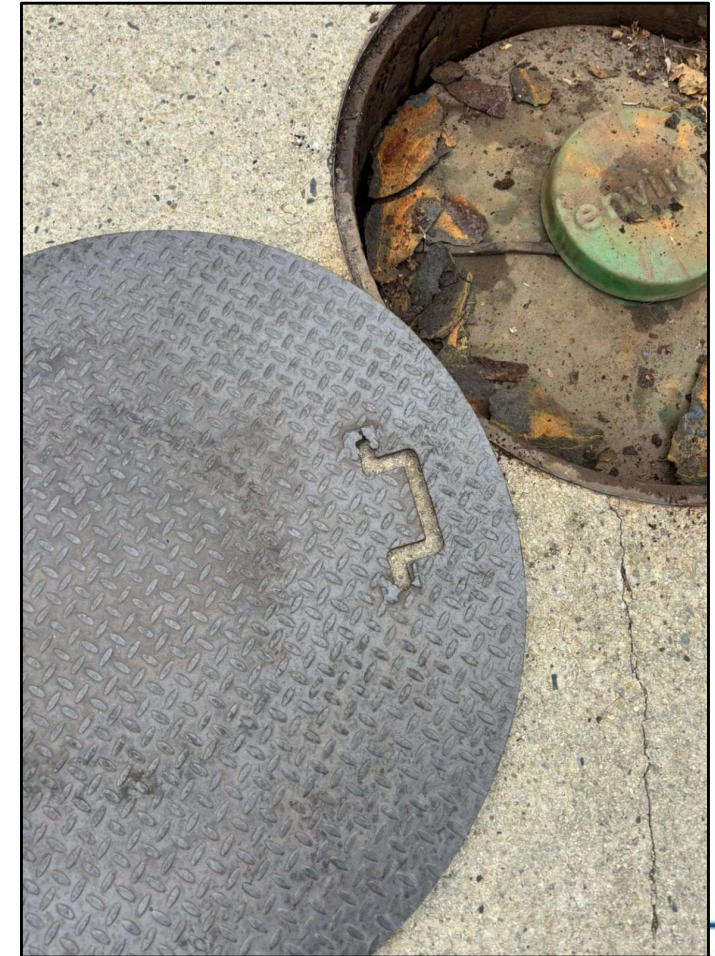
Holes in turbine sump manhole cover, allowing water to infiltrate sump
