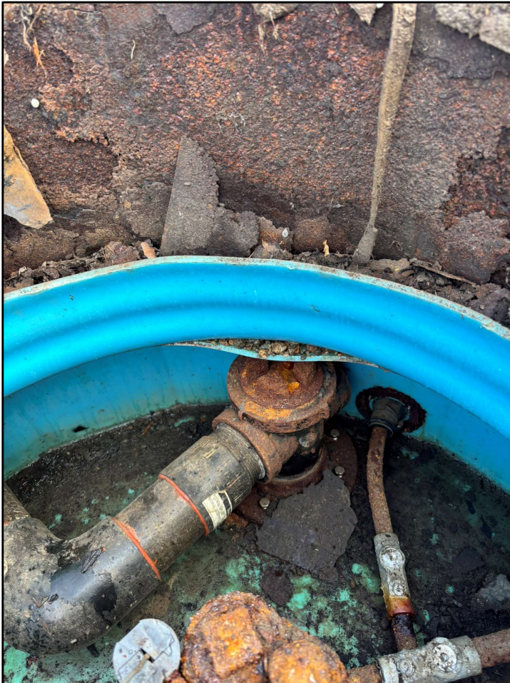
Crack in premium gasoline turbine sump
