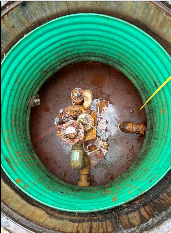
6 inches of water in regular gasoline turbine sump
