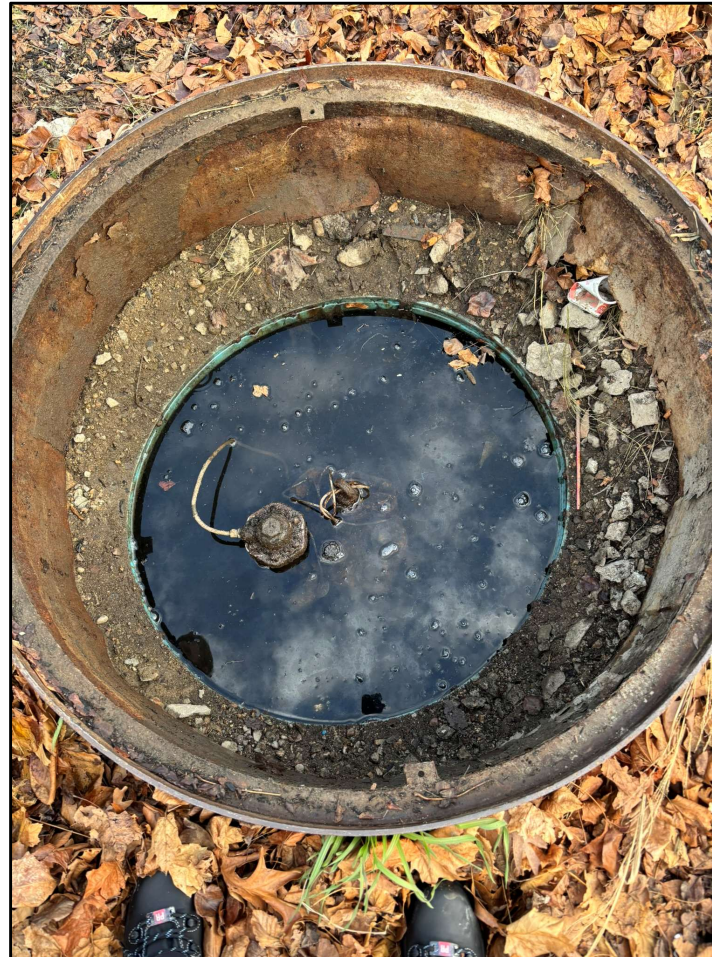
12 inches of water in regular gasoline turbine sump
