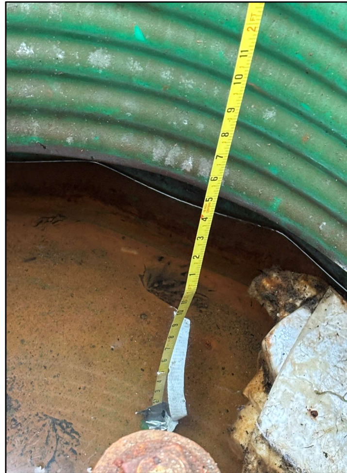
5 inches of water and solid debris in super gasoline turbine sump
