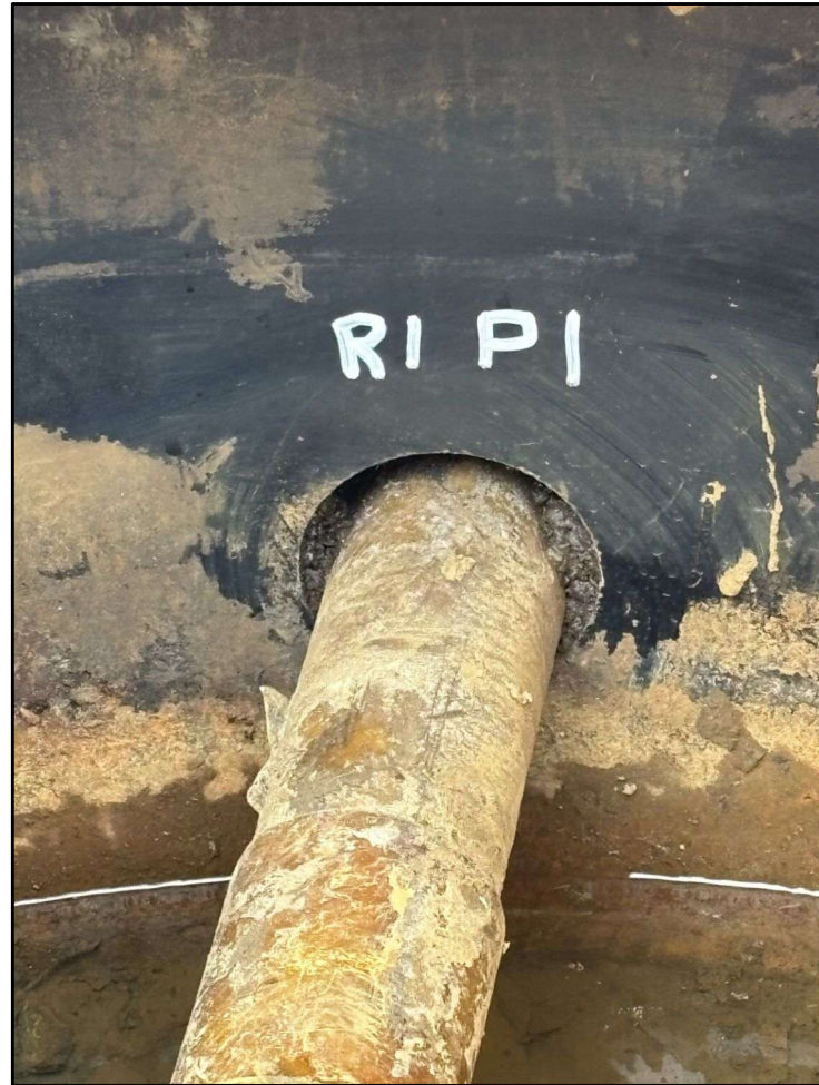
Hole in regular gasoline turbine sump where piping enters
