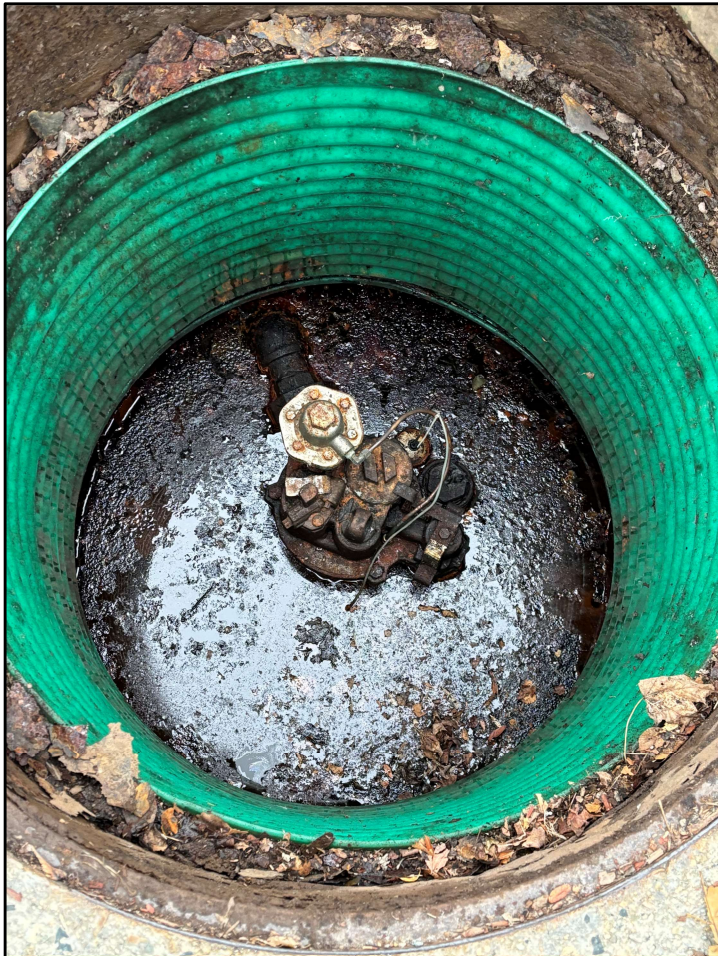
Approximately, 20 inches of water in regular gasoline turbine sump
