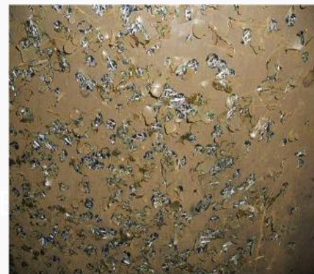
Fiberglass Tank Walls
