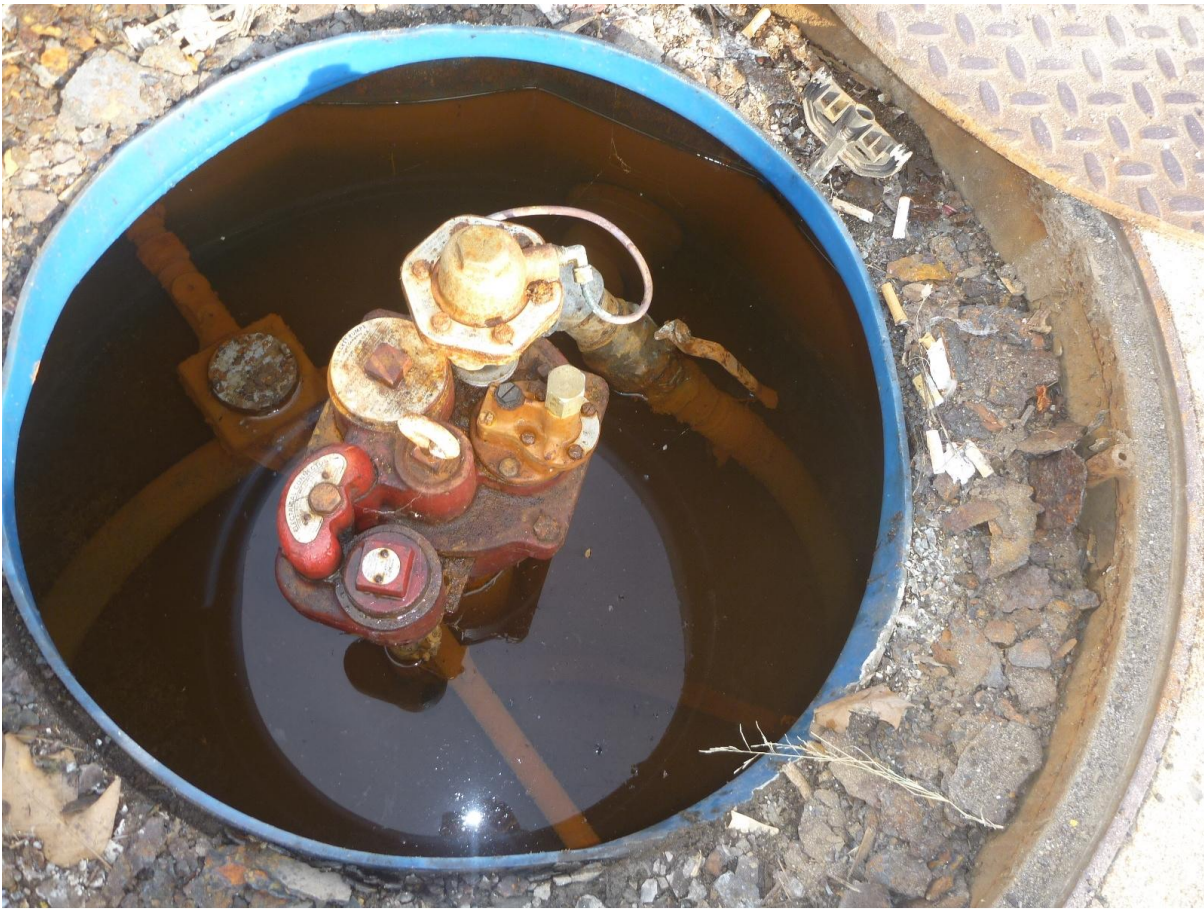
Piping Sump Contains Liquid/Debris - Liquid in tank top pipe sump.
