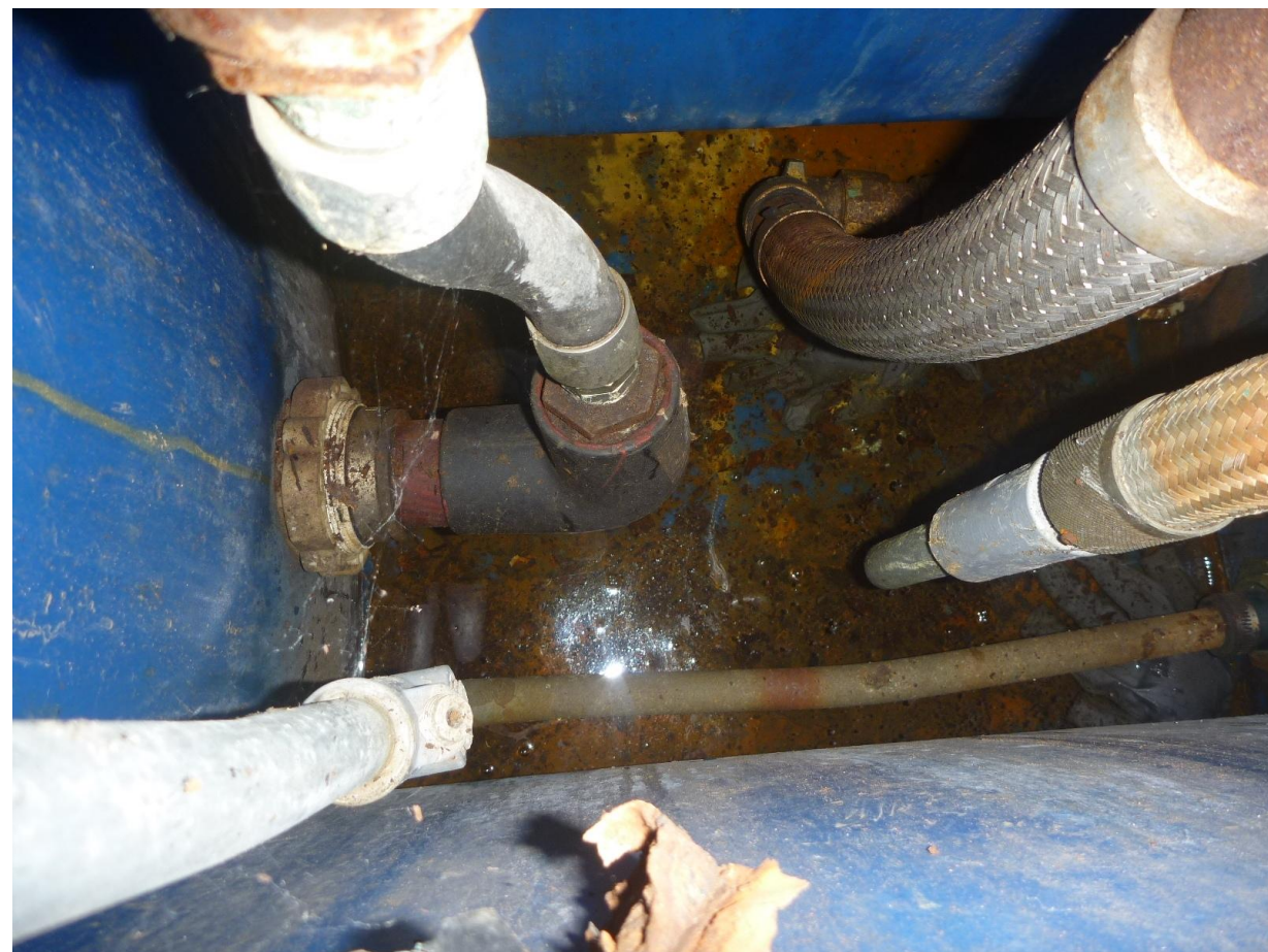
Dispenser Sump Contains Liquid/Debris - Liquid in dispenser containment sump.
