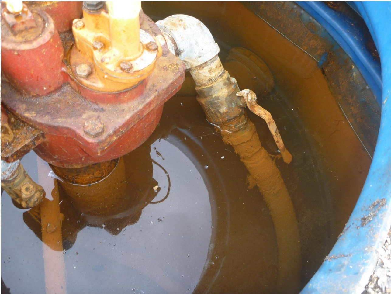
Metal in Contact with Soil/Liquid (at tank top/transition area) - Metal product pipe in contact with liquid in tank top pipe sump.
