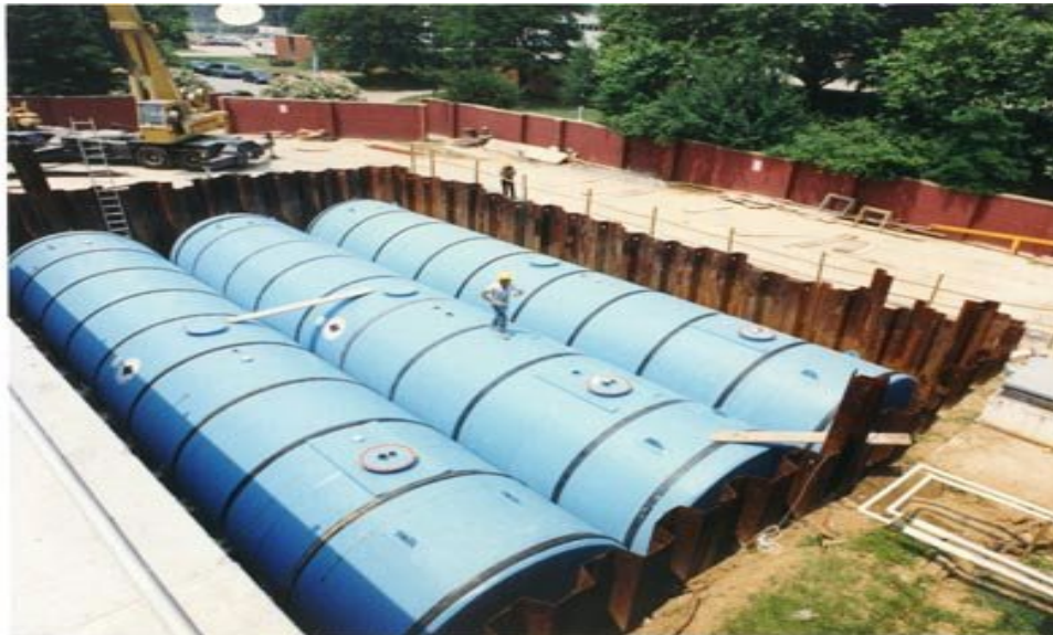
3 Underground Storage Tanks
