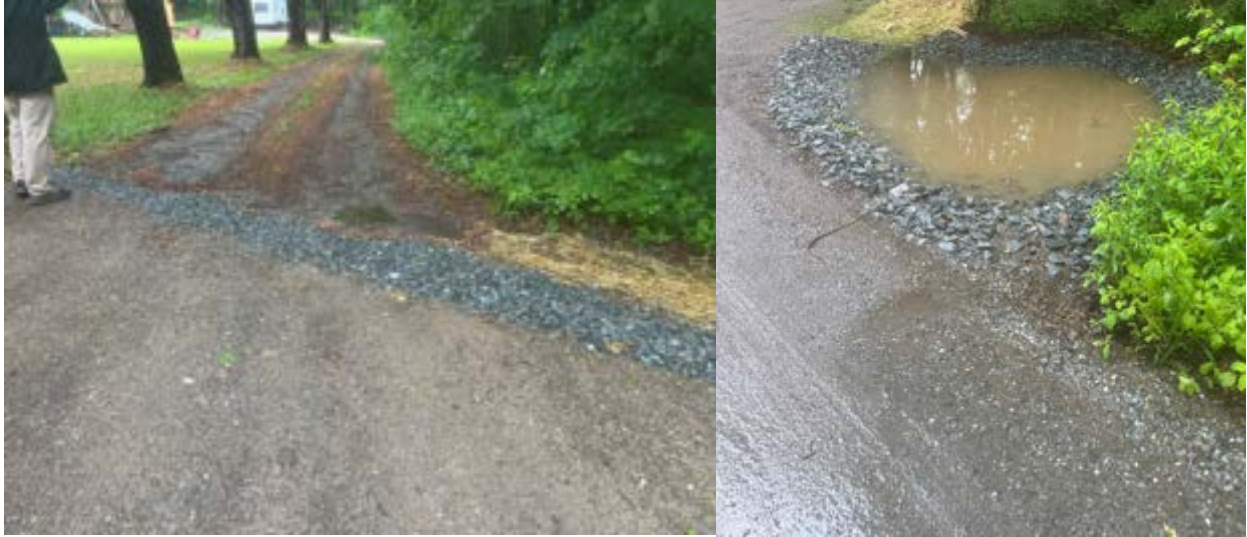
Figure 7. Post construction conditions of the Patton Shore Ledge Drive intersection. To note these photos are after a recent rain storm. Sedimentation basin does not have consistent pooling water.
