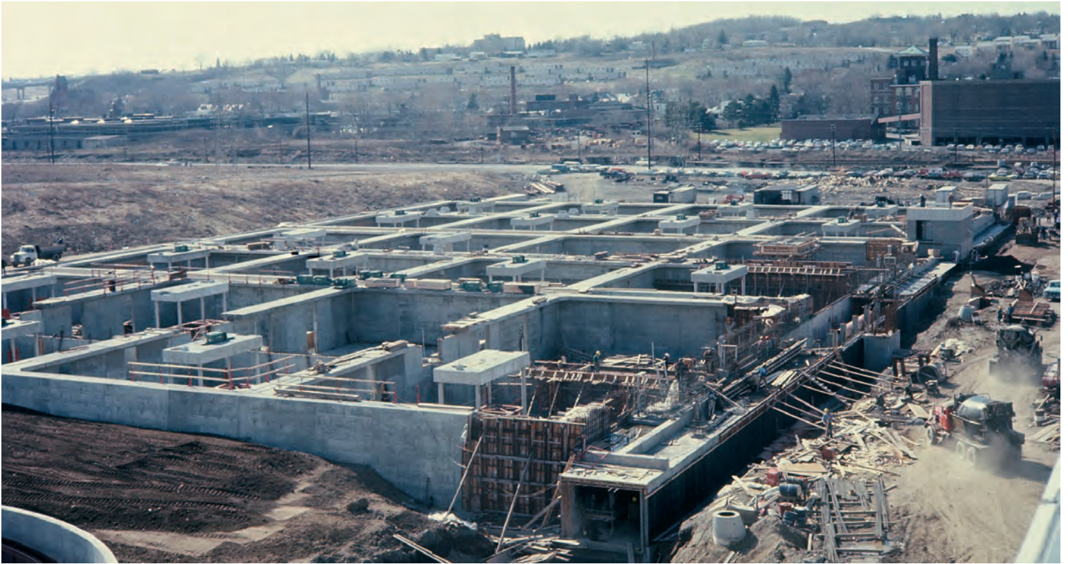
Aeration tanks, North Plant.
