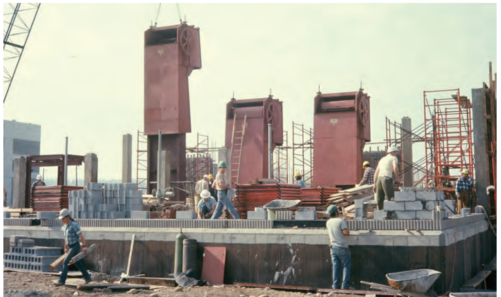
Mechanical fine screen placement, North Plant.
