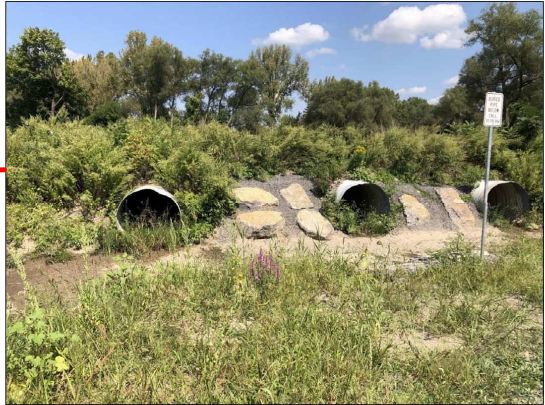
Existing culverts (undersized for current flood events)
