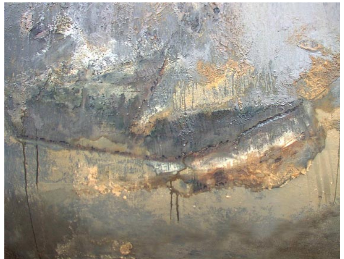
#13 During inspections of excavated USTs we found that damage to the asphaltic or dielectric coating on the outer surface of an UST that occurred during installation could cause preferential corrosion where the bare metal was exposed to the corrosion processes.
