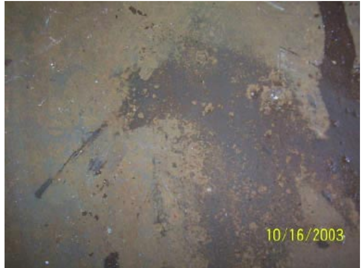
#12 Internal corrosion and pitting.
