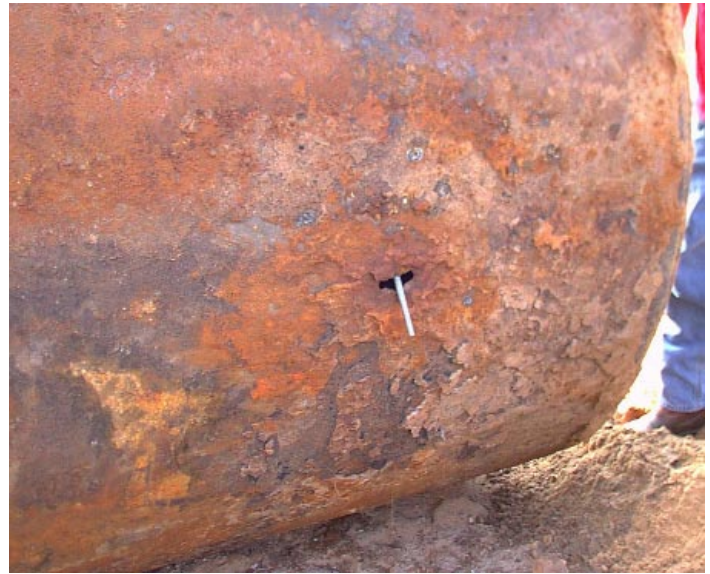
#8 In cases where the non-invasive assessment methodology may have predicted the USTs to be suitable for the installation of a cathodic protection system, it still did not address the need to provide striker plates in USTs to prevent holes being formed under the drop tubes. The non-invasive assessment of this tank predicted uniform corrosion.
