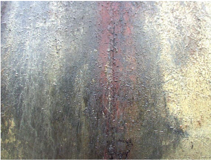
#5 Split weld seam or crack in tank wall.
