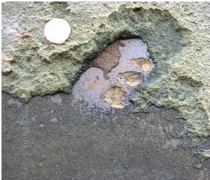
# 1 Potential "rust plugs."
