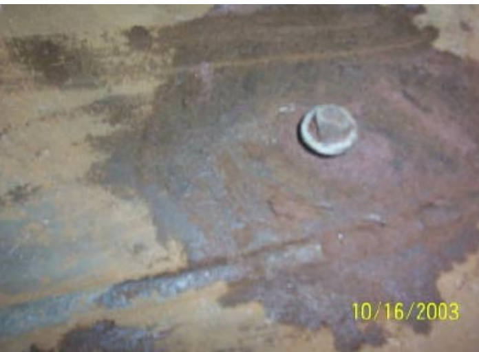
#7 Internal corrosion so severe the tank could not be repaired for lining. The assessment of this tank predicted uniform corrosion.
