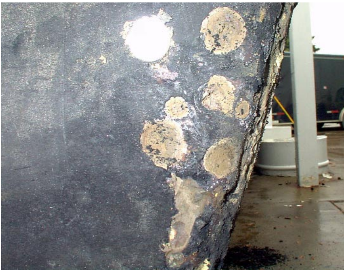
#6 Pitting corrosion and preferential corrosion of the weld seam along the endcap weld.
