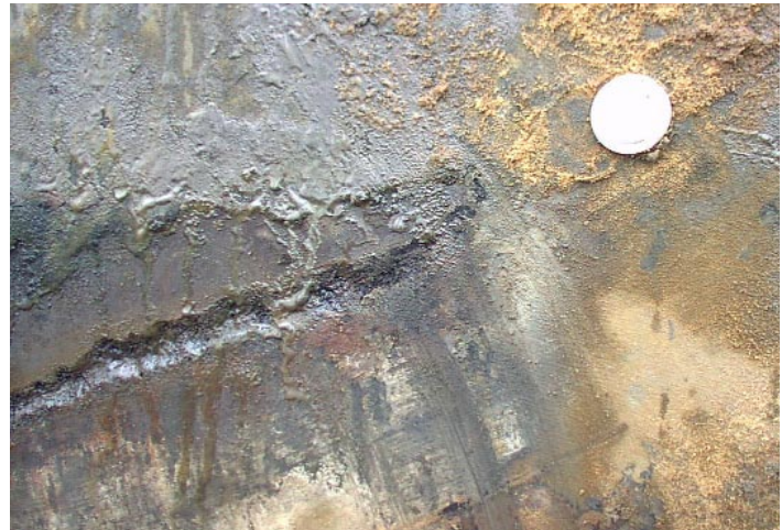
#9 Pitting along damaged area penetrated about 1/4" into the metal. The non-invasive assessment of this tank predicted uniform corrosion.
