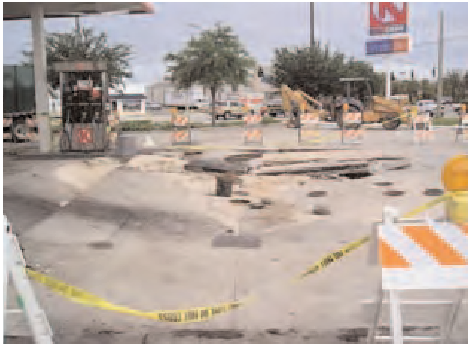
The lightning-impacted site showing subsidence of the tank pad over the UST area.
