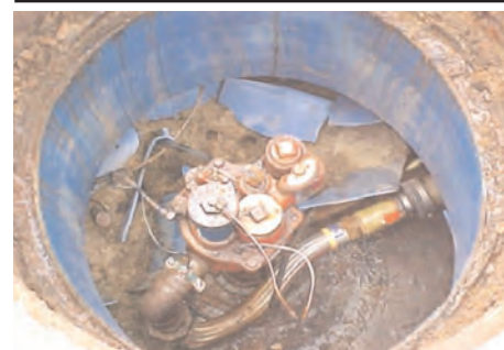
A caved-in, waterlogged tank-top sump.
