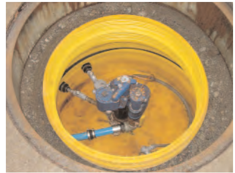
Fairly typical Maine tank-top sump. There is some staining, most likely due to water intrusion, but the sump is now dry. This picture was taken during a random, unannounced inspection.
