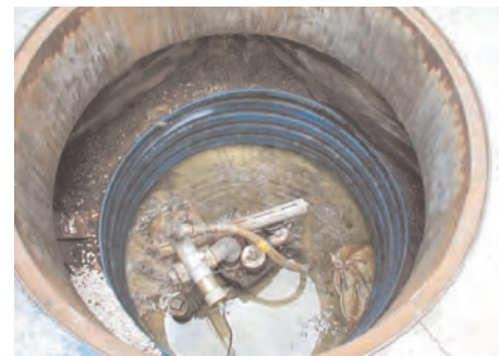
Waterlogged tank-top sump with disabled sump sensor.
