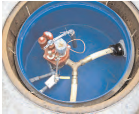
Tank-top sump at an Environmental Leader facility in Maine. Believe it or not, this sump was six years old at the time the picture was taken.
