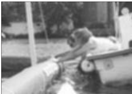
A crew on the Charles River adjusts a portion of the Gunderboom Beach Protection System, which delivered promising results in a study of the system's ability to shield the river's swimmers from high levels of bacteria and pollutants.
