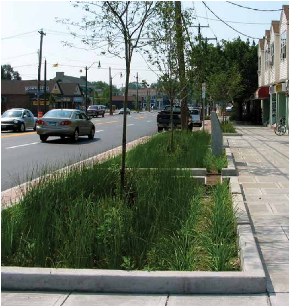
On Main Street in Bridgeport, Connecticut, a linear roadside bioretention basin stands ready to absorb stormwater.
