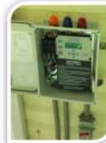
Standard I/A OWTS Control Panel
