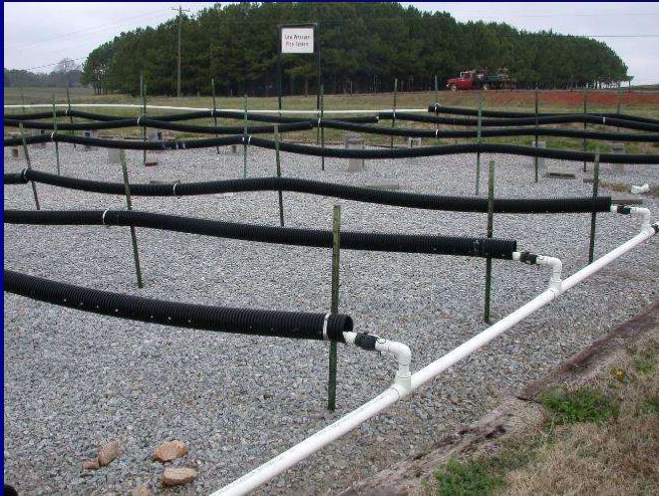
End feed manifold
