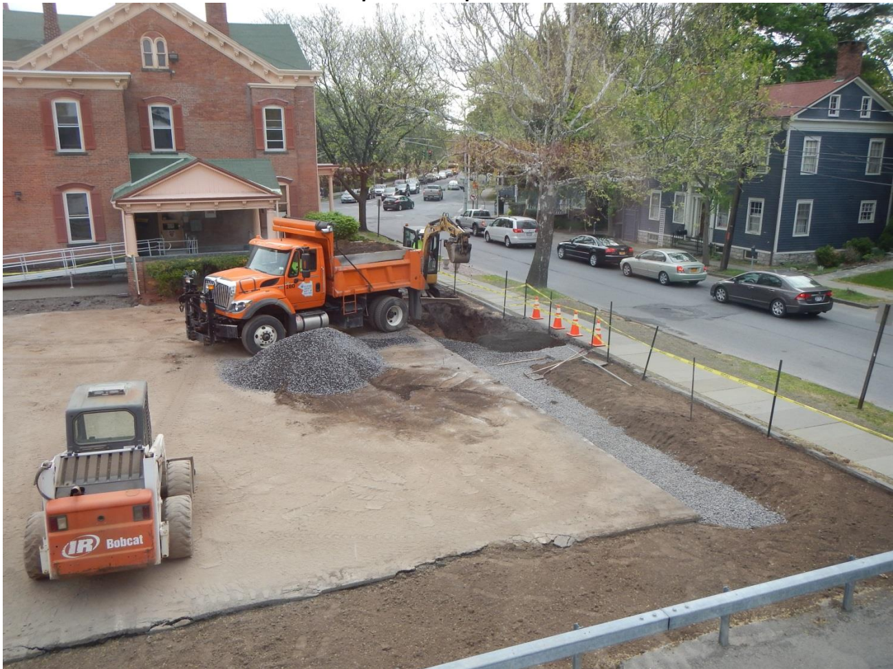
New bioretention soil in planting bed areas in addition to placement of the gravel sub-base underneath the permeable pavers.
