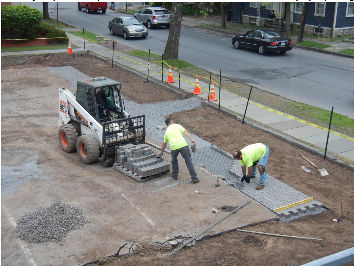
Installation of the permeable pavers between the bioretention areas and the employee parking area
