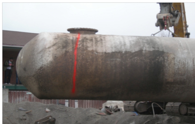
Figure 2. 10,000-gallon double-walled fiberglass UST with red paint on the crack.
