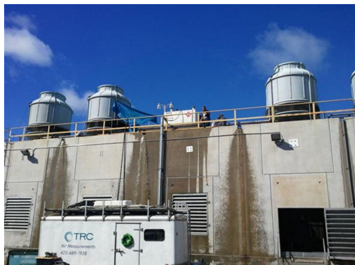
Figure 2. An example of what can happen when a day tank on a building lacks appropriate overflow prevention and tank-rupture controls that would prevent the automatic emptying of the main storage tank onto or into the building. The visible staining on the front of this building is diesel fuel. [Photo Courtesy of Guam EPA]
