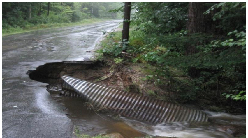
Road washout in Jackson, NH
