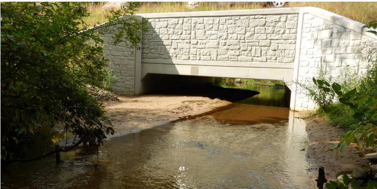
Open-bottom box culvert at McQuesten Brook and Eastman Ave., Bedford, NH – credit: Melinda Bubier
