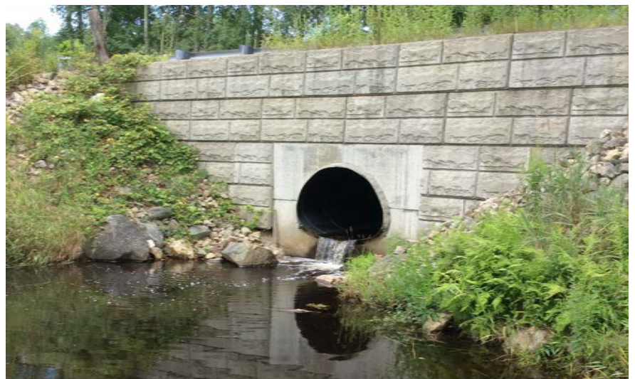
Perched culvert crossing under Ten Rd., Rochester, NH – credit: NHGS
